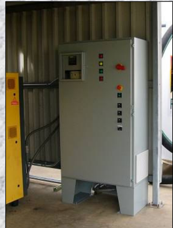
PLC Panel for SVES
