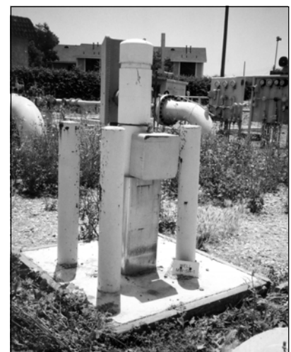
Well MW-SF-4, a vapor extraction well located in the southern area near the Intermediate Block Valve, was used for groundwater monitoring after the release was detected.
