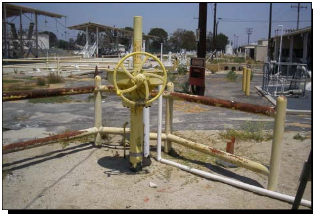
Intermediate Block Valve. Pipeline testing in January detected a small, short-term leak in the southern area. It was immediately repaired, and the remainder of the SFPP pipelines were intact.
