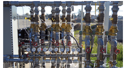
Remediation Piping Controls
