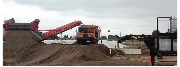
On-Site Soil Treatment System
