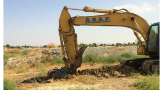
Excavation of contaminated soil at DFSP Norwalk Tank Farm Site. Contaminated soil will be replaced with clean soil
